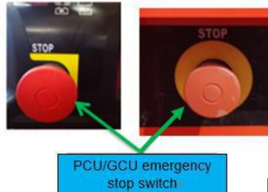
Fig. 9.7 Emergency stop switches of PCU and GCU
