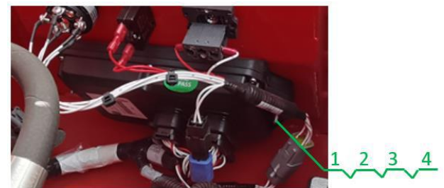
Figure 5.16 Electrical control unit
